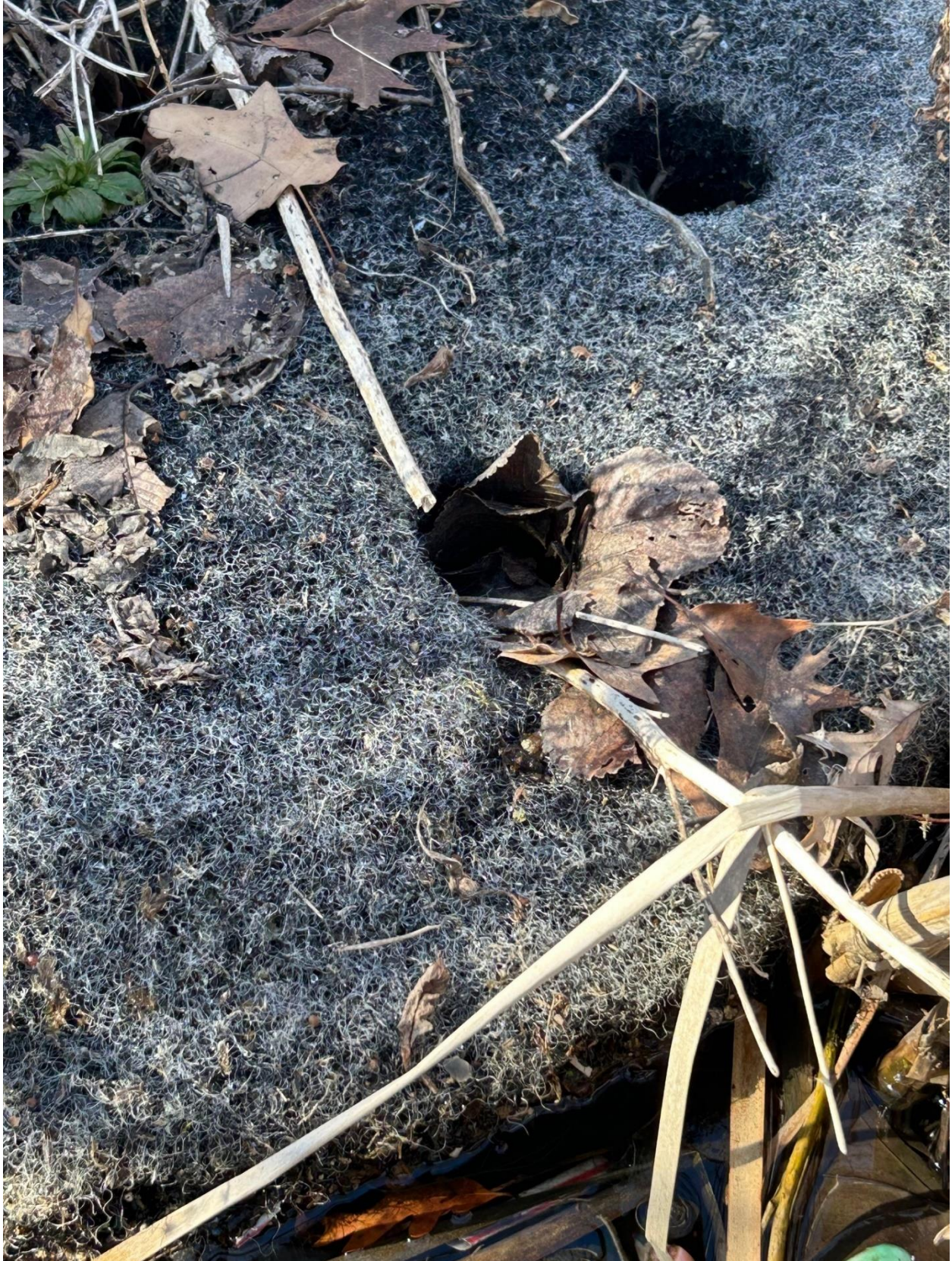
Bleached plastic fibers show evidence that UV protectant is failing.
