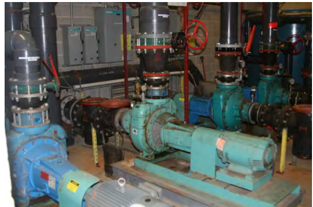
Existing horizontal pumps above water level
