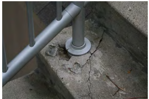
Concrete spalling at slide tower handrail
