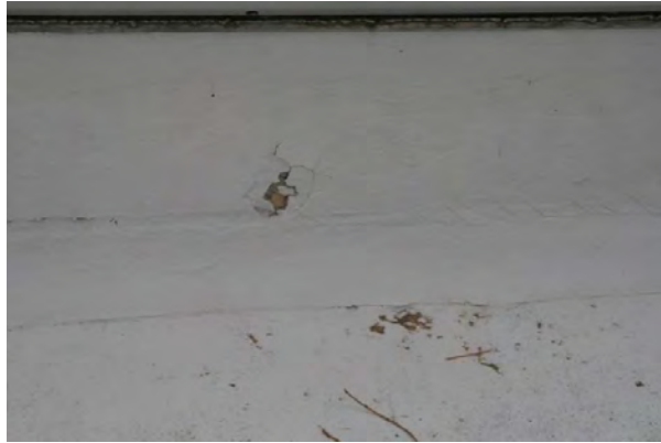
Concrete spalling and deterioration
