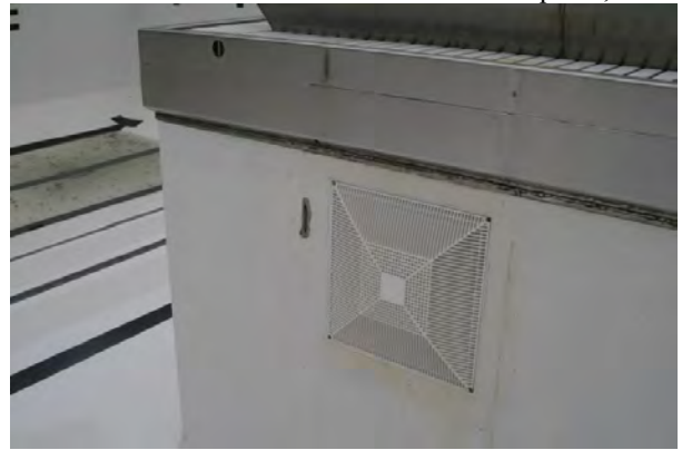
Hole in side wall near grate
