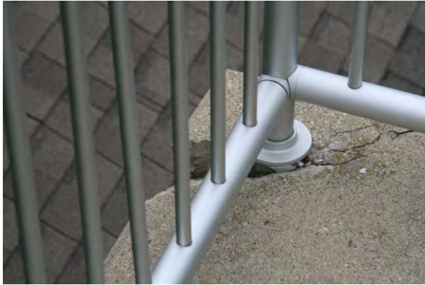
Concrete spalling at corner post of guardrail
