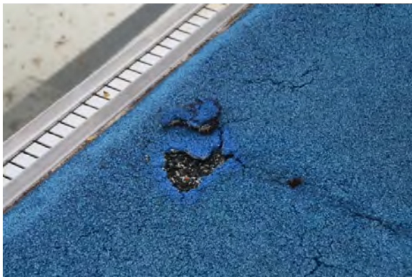
Safety mat deterioration
