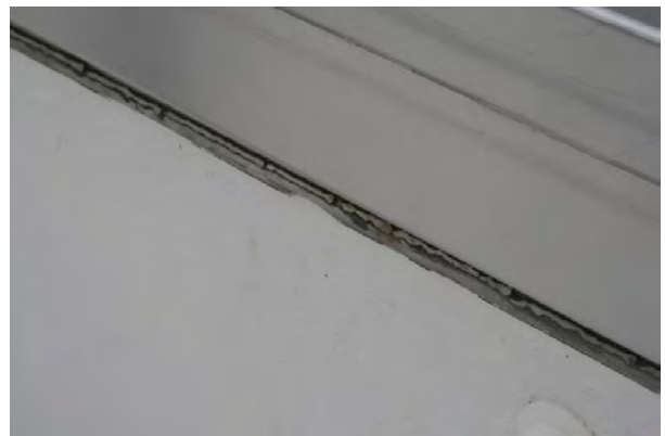
Failed caulking at gutter
