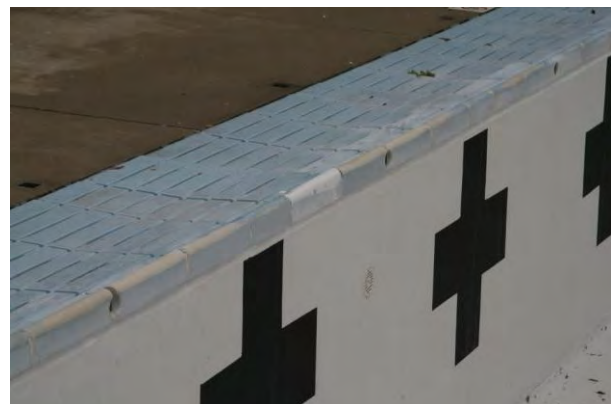
Damaged rim flow coping
