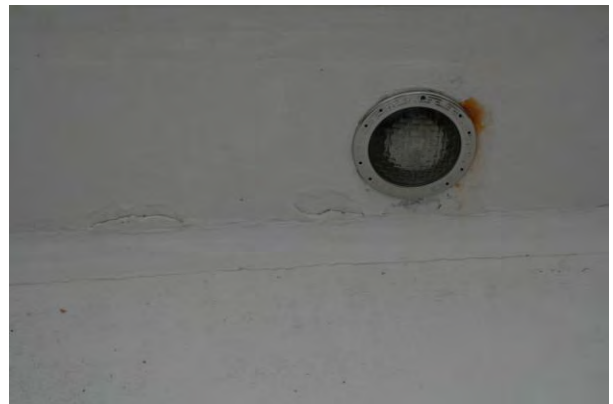
Paint spalling and evidence of water seepage
