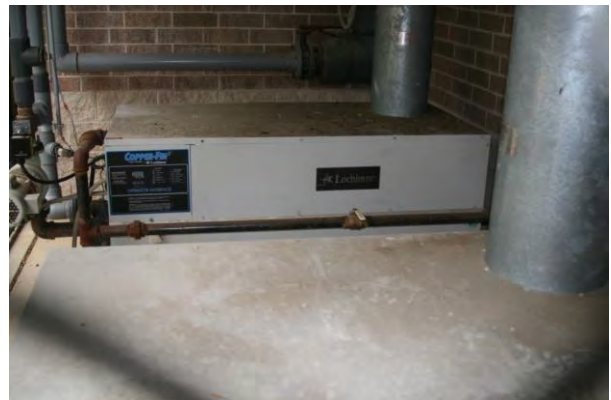
Existing inefficient pool heaters
