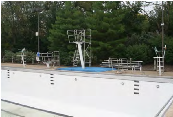
3M board with ladder access
