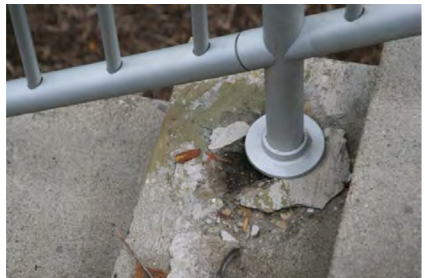
Concrete spalling at slide tower handrail
