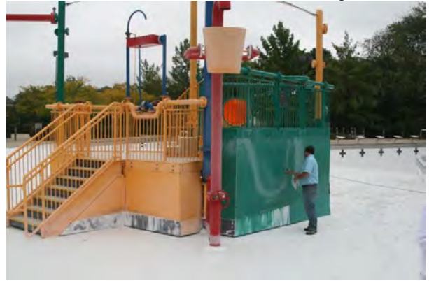
Discoloration on existing climbable feature
