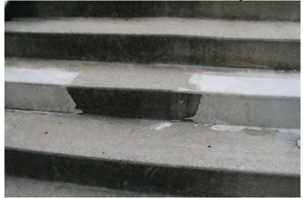
Slide tower stair conditions
