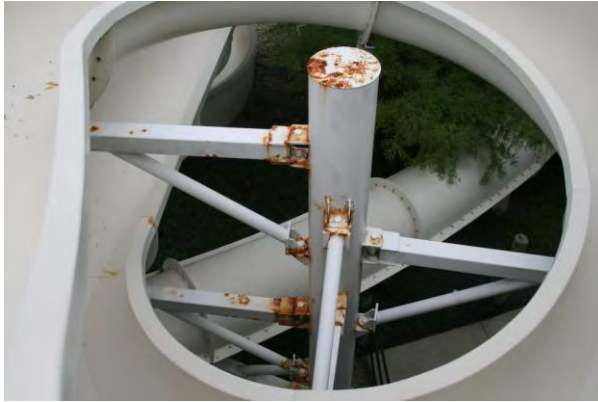
Slide support oxidation
