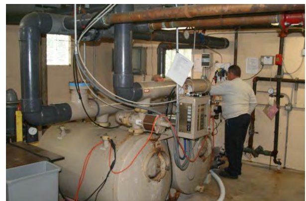
Existing horizontal filters
