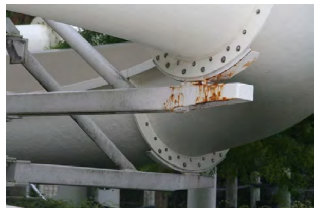
Slide support oxidation
