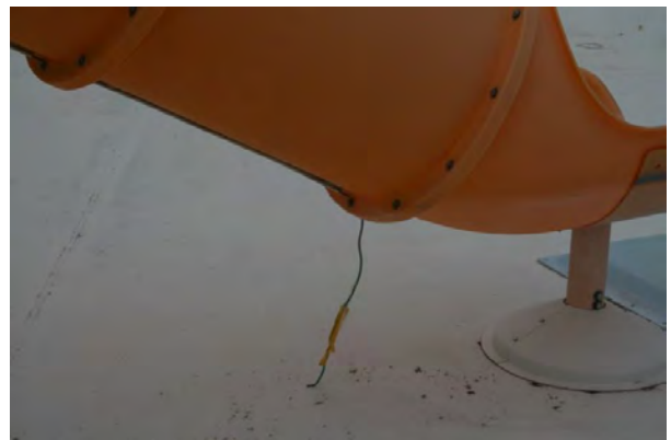
Exposed grounding wire at kiddie slide
