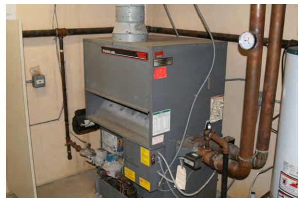
Existing outdated inefficient heater
