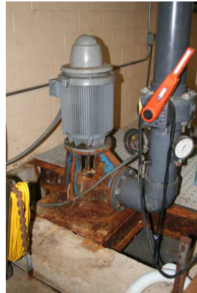
Existing turbine pump
