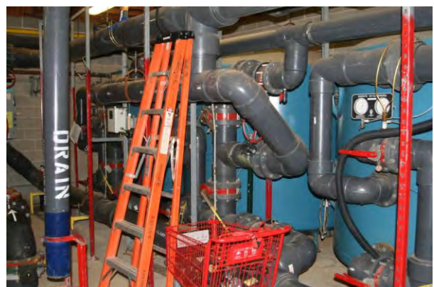
Existing water filtration system
