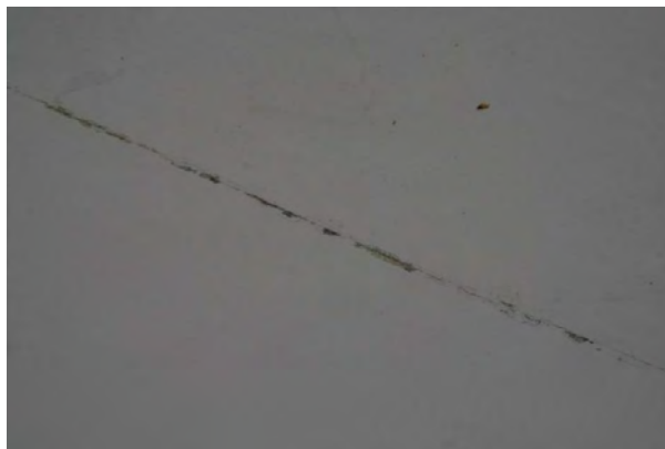
Separation of expansion joint
