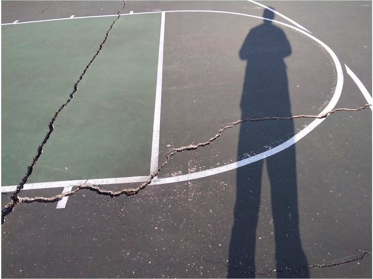
NEWTON PARK BASKETBALL – DISREPAIR
